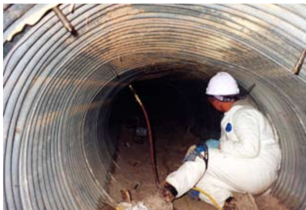
Polyurethane grout injection used to strengthen soil surrounding a stream culvert under Hwy. 50, permeates sands and clays. ---Clifton, CO
