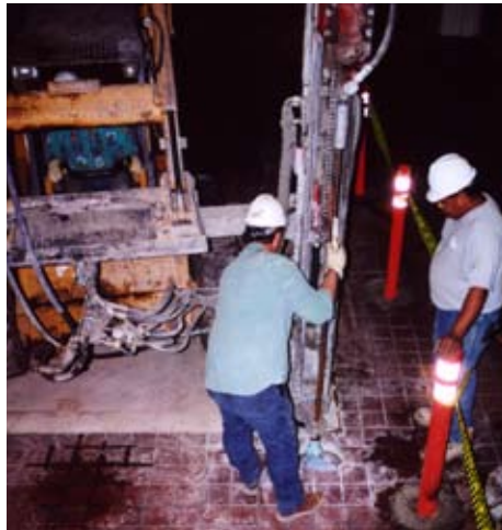
Installing micropiles inside Walker Field Airport terminal for new stairwell foundation. -- Grand Junction, CO.
