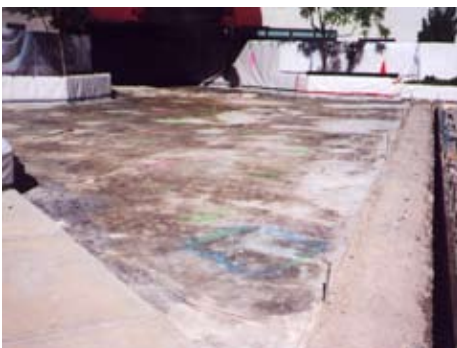
Before: Repair of concrete deck over Parking garage at Horizon Towers. --- Grand Jct. CO.
